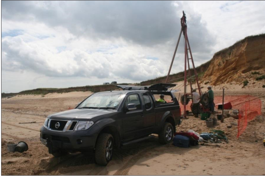
Figure 7 Coring using a cable percussion drilling rig on the foreshore at Happisburgh Site 1, July 2012. Photo by Peter Hoare.
