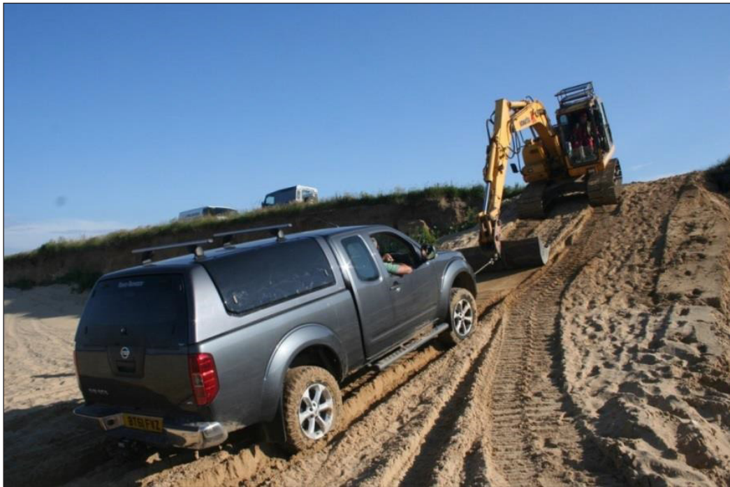
Figure 8 The difficulties of exiting the beach with the cable percussion drilling rig and support vehicle at Happisburgh Site 1, July 2012. Photo by Peter Hoare.
