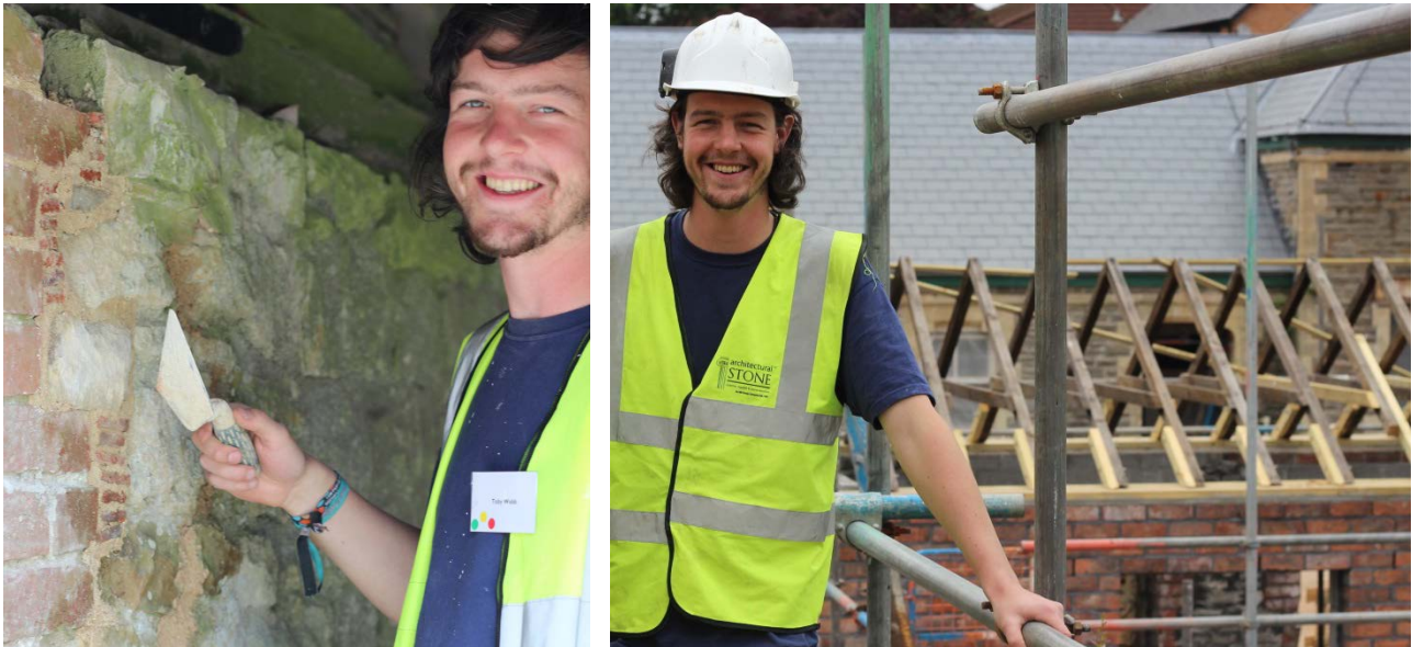
TOBY MAKING A TILE REPAIR ON THE SPAB WORKING PARTY 2015 (LEFT) ON SITE AT INSOLE COURT (RIGHT)
