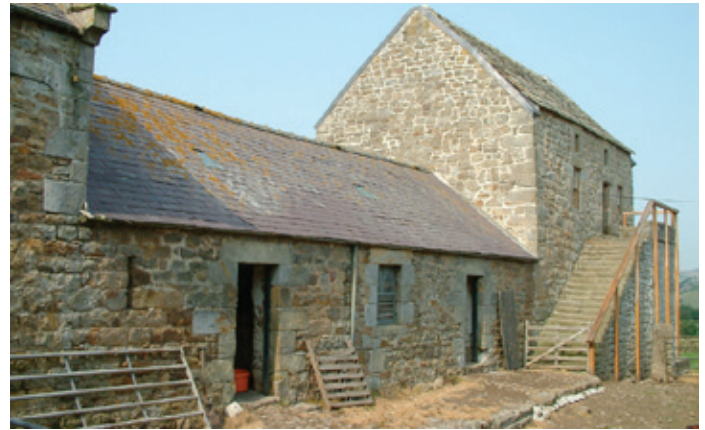
Cow house attached to a bastle near Bewcastle in Northumberland. Note the raised causeway to enable dry access, the ventilation slit to the left, and the part-glazed window to the right set in an opening widened in the mid-late 19th century. Photo © Jen Deadman
