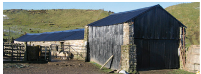
A single-storey shelter shed and (in the foreground) an attached hay barn in Lunedale, North Pennines. © Jeremy Lake
