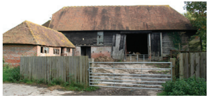
17th century combination barn with integral stable and attached 19th century shelter shed for cattle in the High Weald. Photo © Bob Edwards
