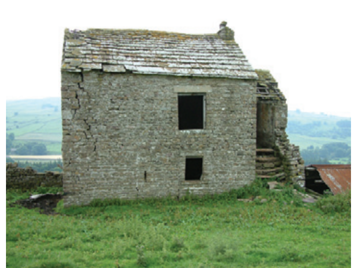
A small-scale early 19th century example in Weardale. Such buildings were commonly extended in linear fashion. Photo © Jen Deadman
