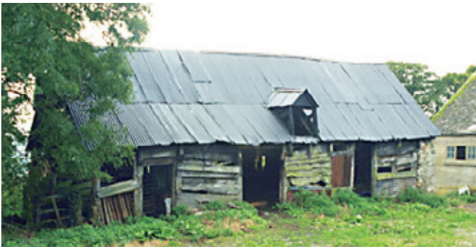
Single-storey timber-framed cow house in the Shropshire Hills, of a type found along both sides of the border with Wales. Photo © Jeremy Lake
