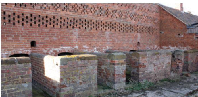
Pop holes to a hen house above a pigsty in north Shropshire, an unusually decorative arrangement. Photo © Jeremy Lake
