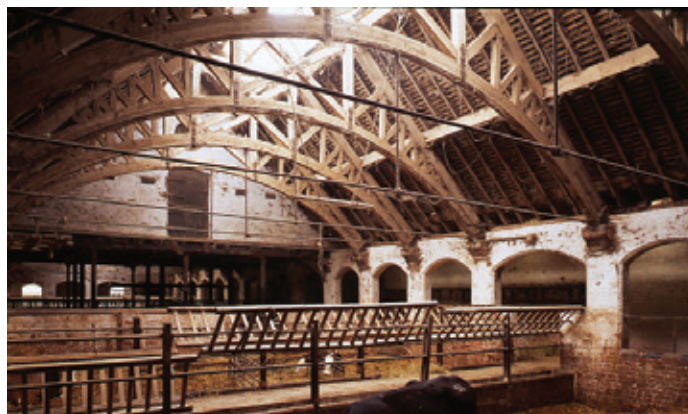
The interior of a covered yard within a planned farmstead at Apley Park in Shropshire, listed at grade II*. The roof makes use of laminated timber. The park was purchased in 1867 by William Orme Foster, an ironmaster from Stourbridge. The building was built to the designs of local architect Robert Griffiths (1825 – 1888) and incorporated a great deal of technical innovation such as the use of steam power for threshing and processing feed. Photo © English Heritage/Mike Williams
