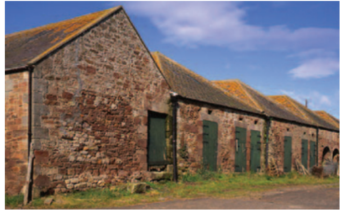
Range of loose boxes marked by their individual doors in a large planned farmstead on the coastal plain in Northumberland. Photo © Mike Williams/ English Heritage
