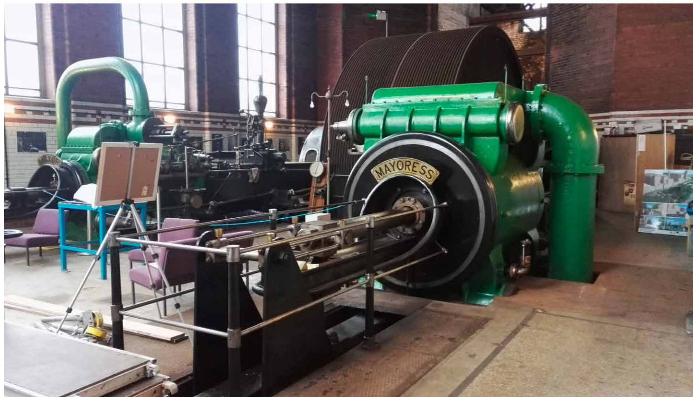
Above left: The horizontal cross-compound steam engine that survives in-situ at Leigh Spinners Mill within the recently repaired engine house. © University of Salford
