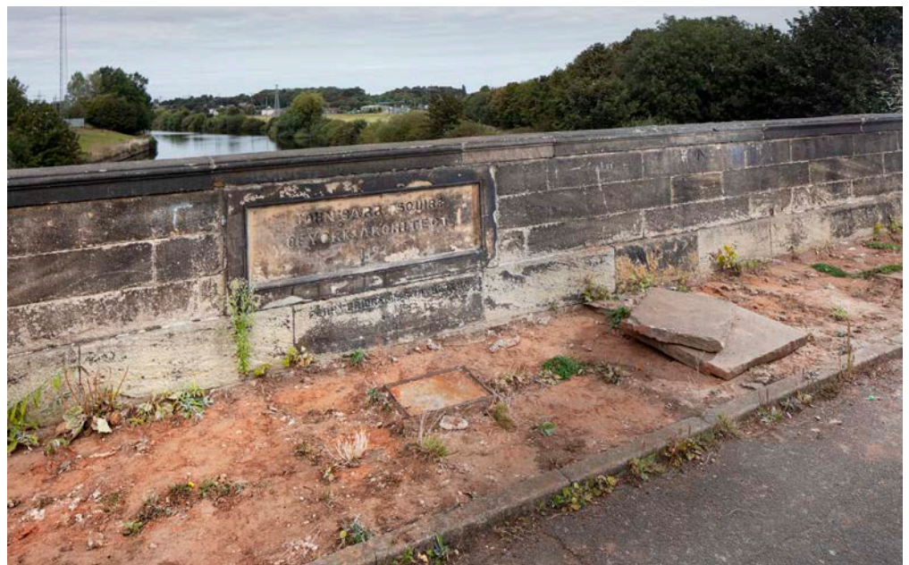
Figure 1: Ferry Bridge, Old Great North Road, Brotherton, Ferrybridge, Selby, North Yorkshire. This Grade I Listed bridge by the noted architect John Carr was subject to the theft of paving slabs. © Historic England
