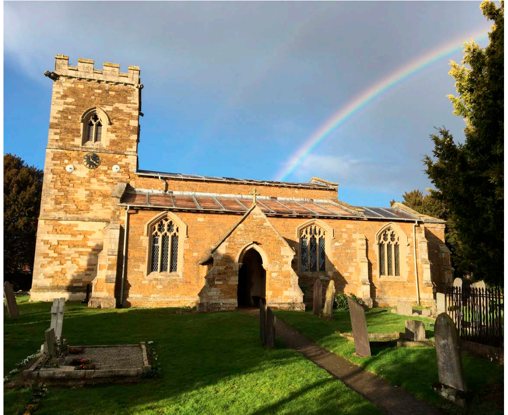
Figure 3: Although not immediately apparent, the lead has been stolen from the roof of this church. © Simon Headley
