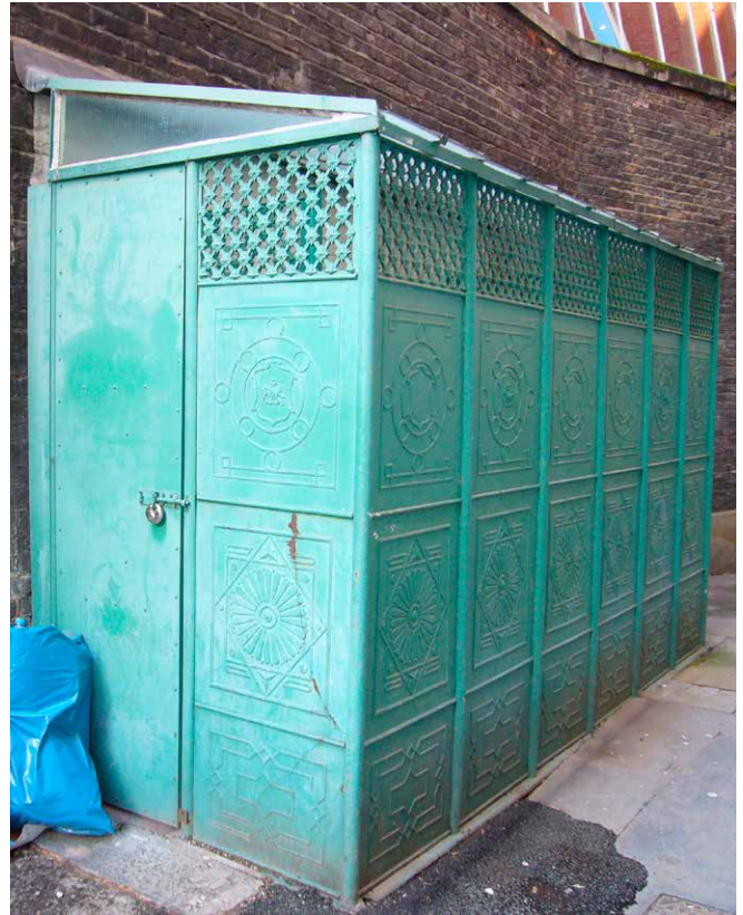
Figure 9 A probably late nineteenth-century cast iron urinal in Star Yard, off Chancery Lane in London’s legal district, manufactured by McDowall Steven & Co of the Milton Iron Works, Glasgow. Listed Grade II.
