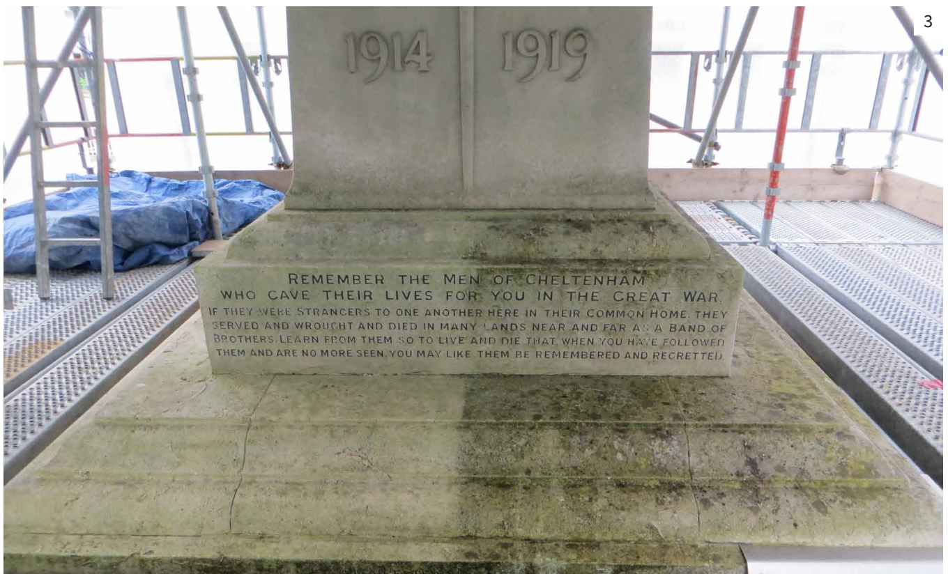
3 The left hand side of the memorial has been cleaned using super-heated water.
