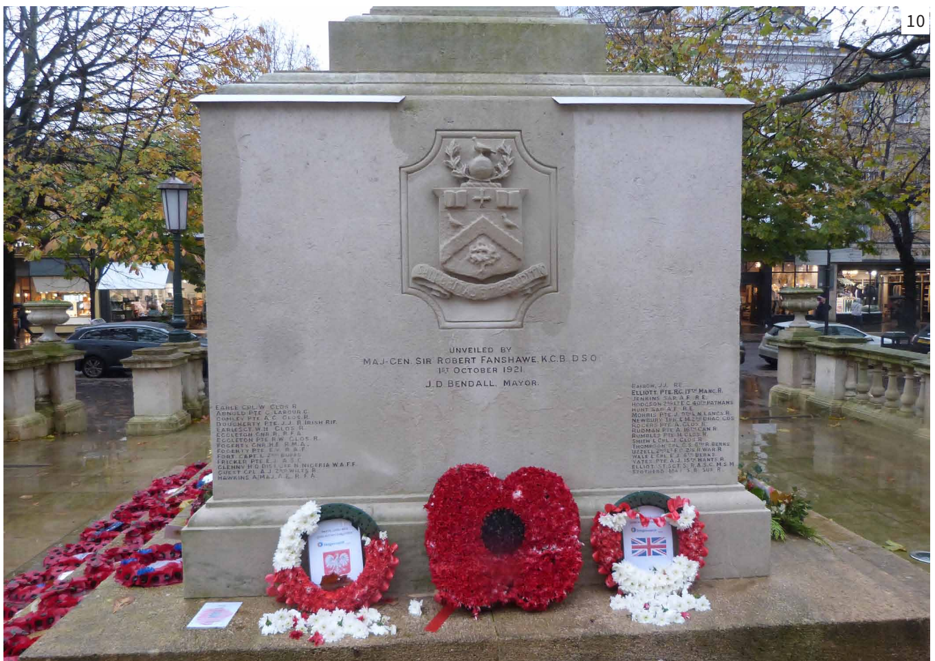
10 West side after completion, with flashing in place. The upper areas of the memorial are developing surface algae after only a few months.
