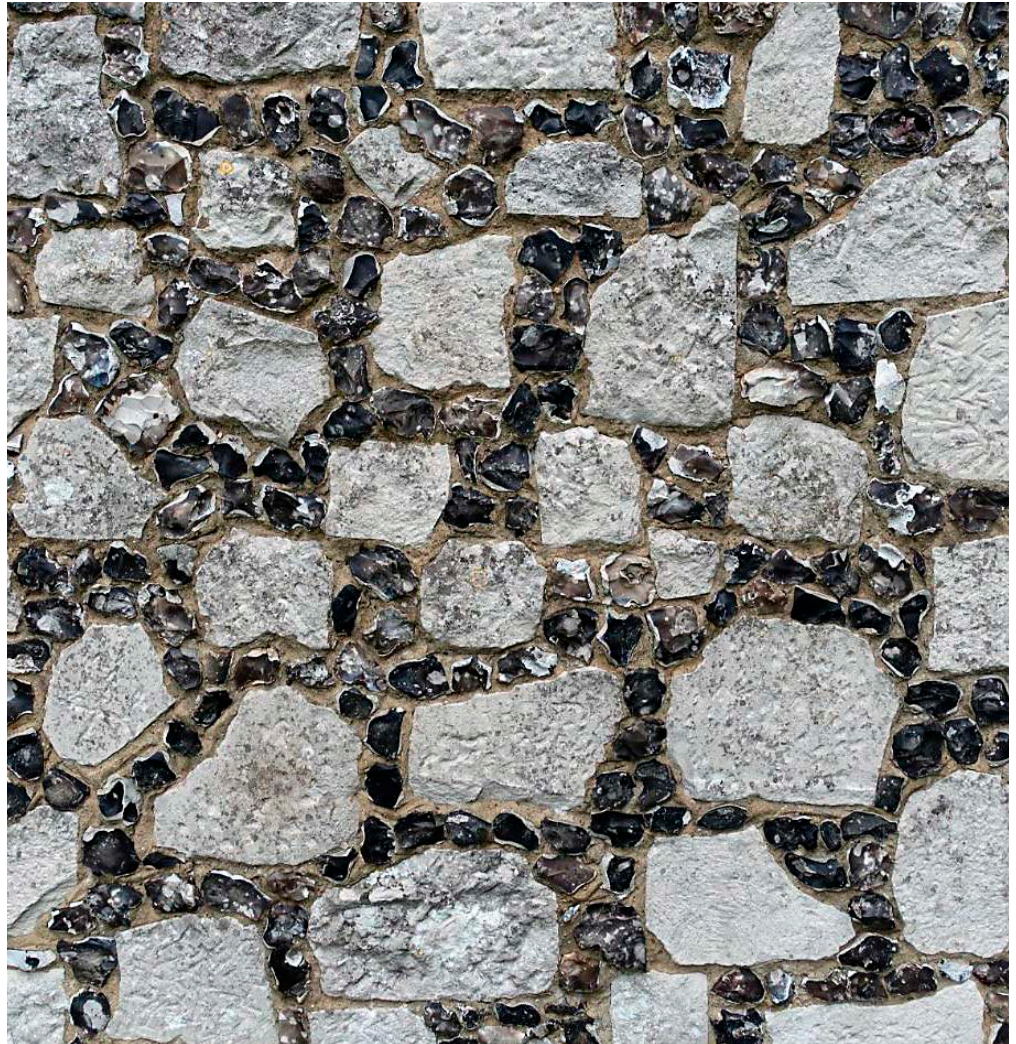
Figure 41: Detail of wall, Church of St Peter and St Paul, Medenham. Chalk block and Quarry Flint.
