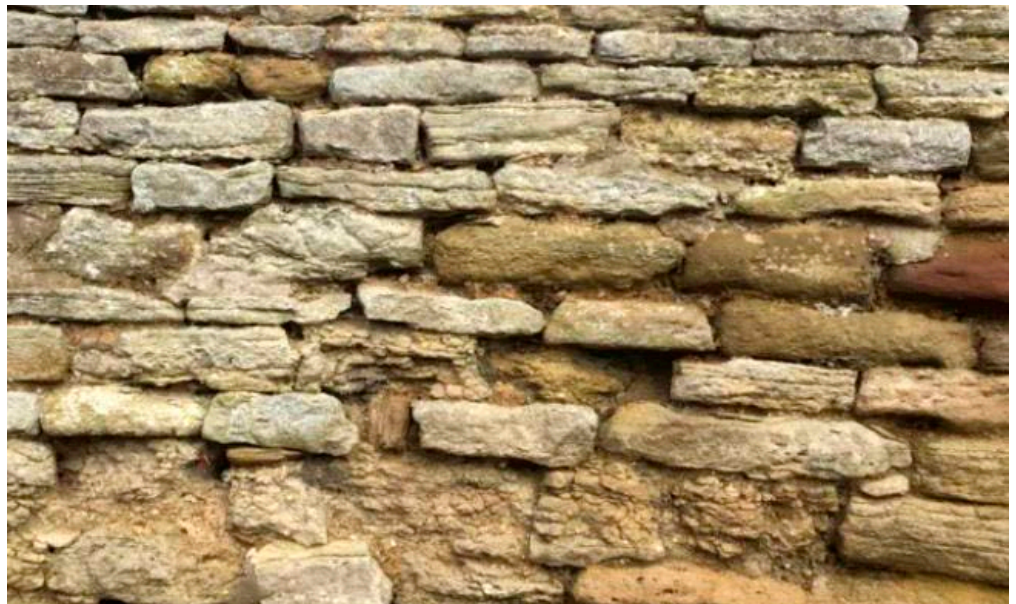
Figure 22: Churchyard wall, Ravenstone. Forest Marble and Cornbrash with Blisworth Limestone and ironstone.
