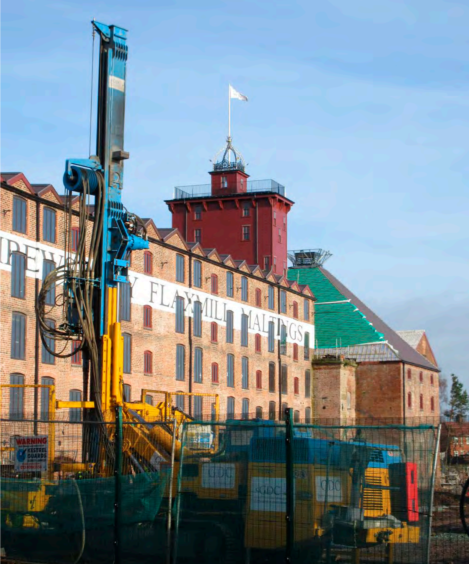
Shrewsbury Flaxmill Maltings is a major renovation project for Historic England, now partly complete and occupied. The Mill (Grade I listed) was a pioneering iron-framed building and it is to be heated in the same progressive spirit. The rig in the photograph is penetrating the ground to a depth of 187 metres to form one of ten boreholes to tap the ground heat for two ground-source heat pumps located in the Main Mill. There is room for more boreholes if this proves the best way to heat the residential development yet to be designed and built on the rest of the site. [Nick Hill, © Historic England]
