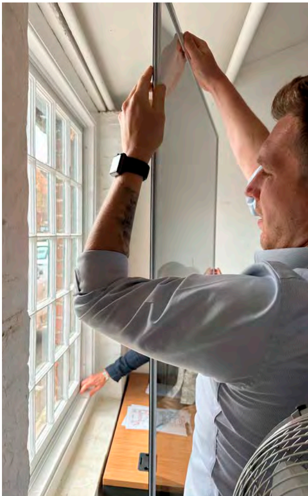
Secondary glazing samples installed in the Works Yard at Hampton Court Palace as part of a series of energy efficiency improvement trials, exploring a number of different options in various locations alongside a data-gathering exercise to establish the most effective solution for a wider roll-out. [© Historic Royal Palaces]
