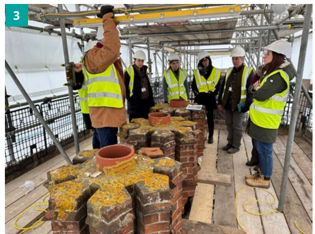
Image 1: The poor condition of the chimney bricks and mortar was discovered during maintenance work nearby, giving the opportunity to see the chimneys more closely. Image 2: Camilla Finlay, HRP Trustee and Architect, visits site with Emma Simpson to see project progress. Image 3: Project Team discuss the chimney condition prior to works commencing. © Historic Royal Palaces
