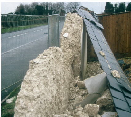
A chalk cob wall had been rendered with an NHL 3.5 render, trapping moisture inside the cob which led to its collapse. (Photo: Kevin Stubbs)
