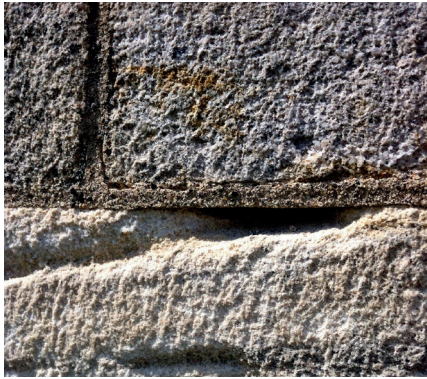
18 years after being repointed in NHL 3.5 mortar, this sandstone is decaying while the pointing remains intact. The mortar is not acting sacrificially to protect the stone. (Photo: Sam Baxter)
